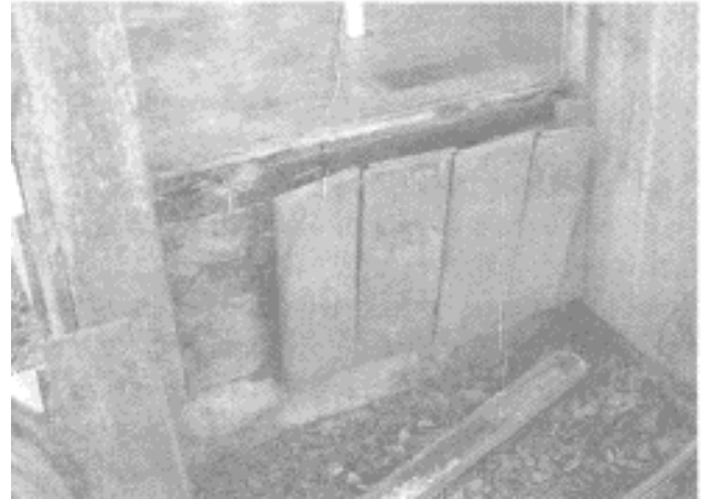
Figure 11. Decay caused by Poria.
