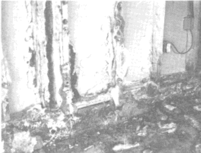
Figure 10. Decay caused by Poria.
